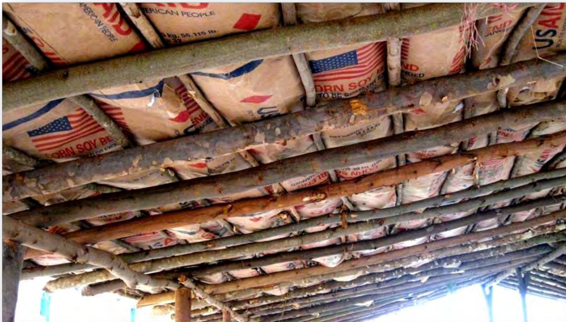
Roof with empty CSB bags - Branding & Marking!
