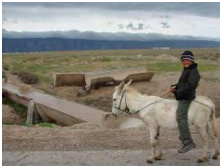
A boy on mule poses next to a damaged irrigation canal that feeds into the irrigation network of WUA “Yangi Hayot” (Jilikul District).
