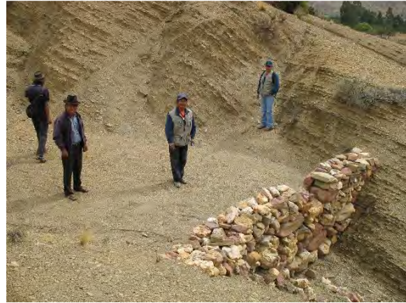
This check dam silted up completely in one year. Powerful object lessons like this help convince communities that soil erosion is real.
