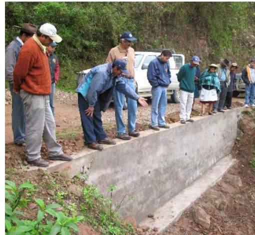
A retaining wall holds the road in place. Most of the structures were well made.
