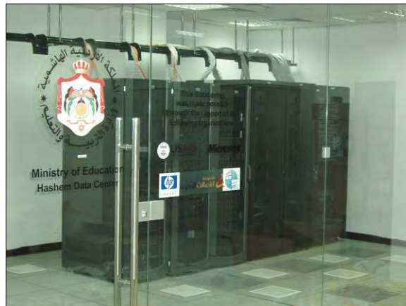
Exhibit 2 The Ministry of Education data center co-located at the Jordan Telecom Hashem Data Center.
