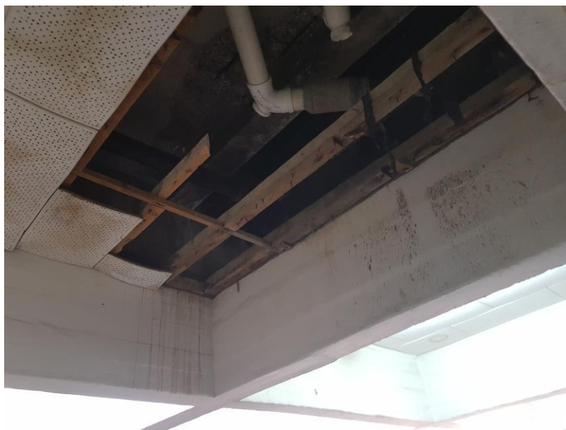
FIGURE 10. CEILING LEAK AT A COE/SOE
