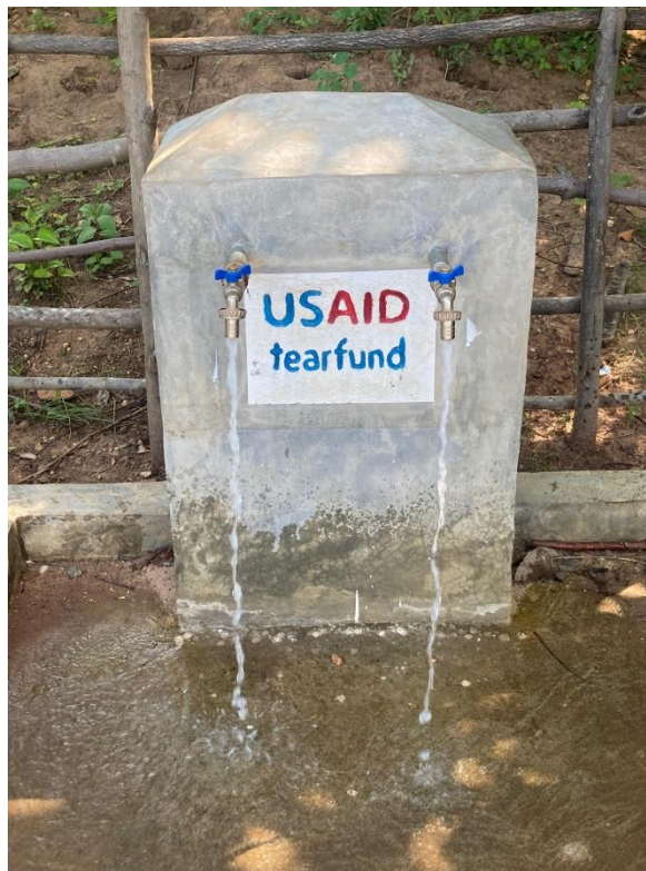
Tapstand in South Kivu
