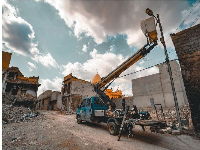
Teams from the General Company of Northern Electricity Distribution (GCNED) install streetlights in West Mosul. PHOTO: IRP I/Chemonics
