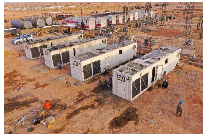
Five generators were repaired at Rutba Diesel Power Station, providing a more consistent supply of electricity to an estimated 25,000 residents. PHOTO: IRP I/Chemonics
