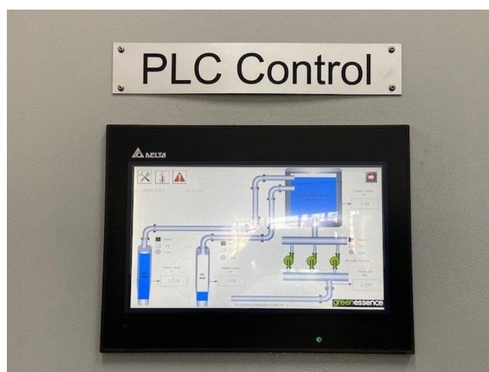
Figure 9. Control at Ghazzeah pumping station
