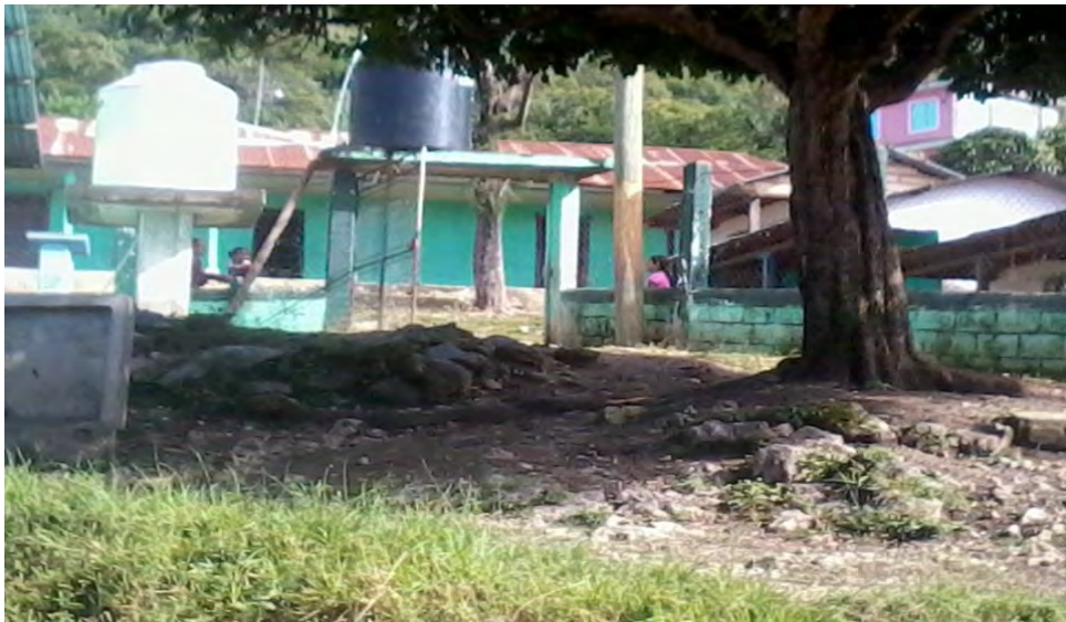
Water storage tank for the school in the village of La Laguna, municipality of San Pedro Necta. Received as a donation and with community collaboration.
