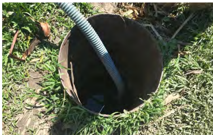
Water pump in Ermera
