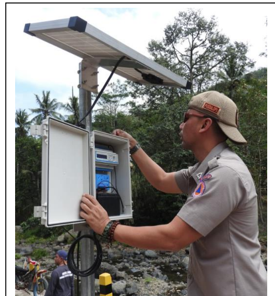
Flood Early Warning System equipment, Sitarjo Village, East Java. Photo: © USAID-APIK
