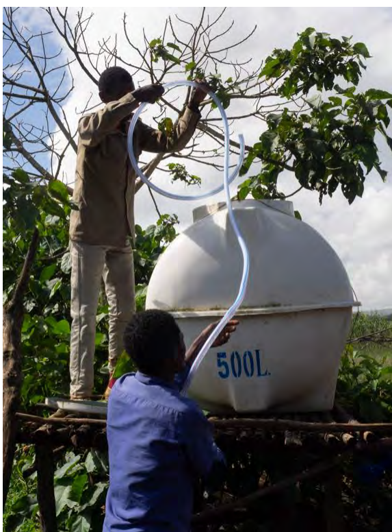
Water drawn from shallow wells using the Magipump is stored in 500 litre tanks for delivery via the drip irrigation system
