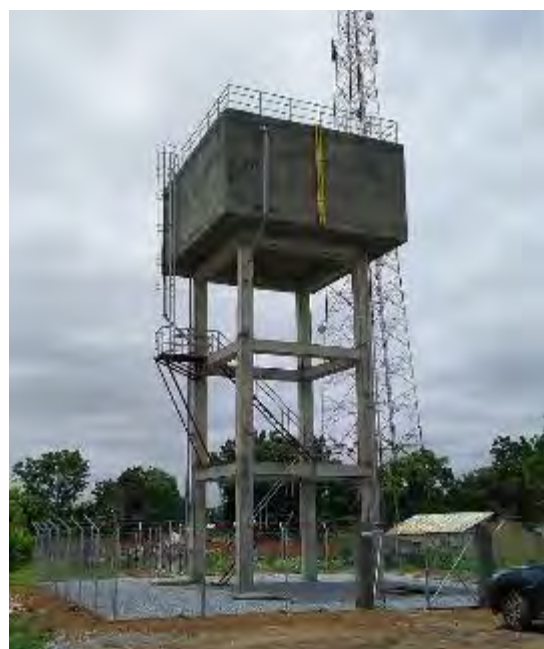
Photo 6: Water tank in the Tuna system
