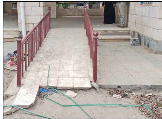
ACCs IDENTIFY REHABILITATION NEEDS LIKE REPAIRING SCHOOL STRUCTURES IN ZENJUBAR COMMUNITY, ABYAN GOVERNORATE
