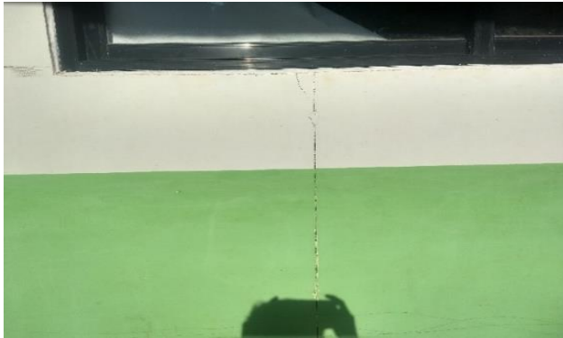
Nepal: Opportunity Village, open joint at exterior wall panels (prefab), Image by IMC staff, 2018
