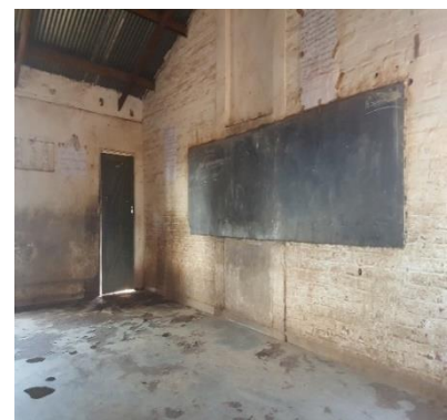
Malawi: Nkomadri Schol, 1980s building in good condition (conventional), Image by IMC staff, 2018
