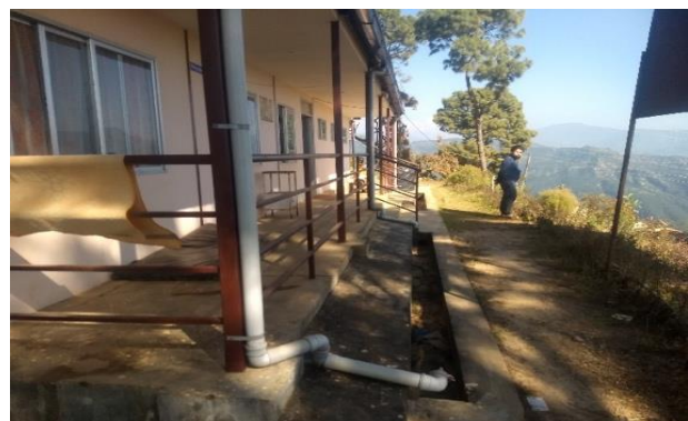
Nepal: GTZ Facility drainage (prefab) Image by IMC staff, 2018
