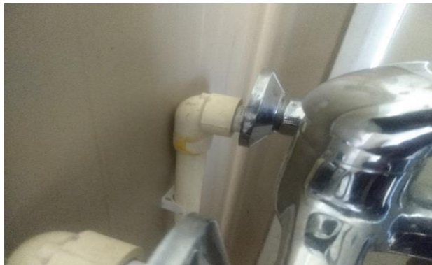
Nepal: Opportunity Village, poor plumbing installation (prefab), Image by IMC staff, 2018
