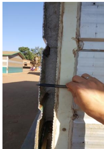
Malawi: Tsbango I Schools, wall panel failure and missing corner flashing (prefab), Image by IMC staff, 2018
