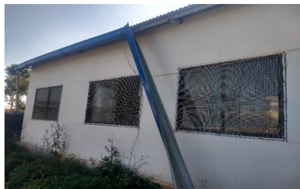
Nepal: Opportunity Village, deficient gutter installation (prefab), Image by IMC staff, 2018
