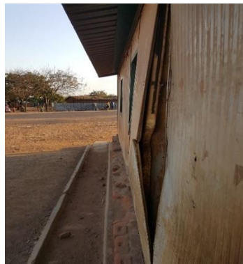
Malawi: Mvama School, failure of wall panels (prefab), Image by IMC staff, 2018
