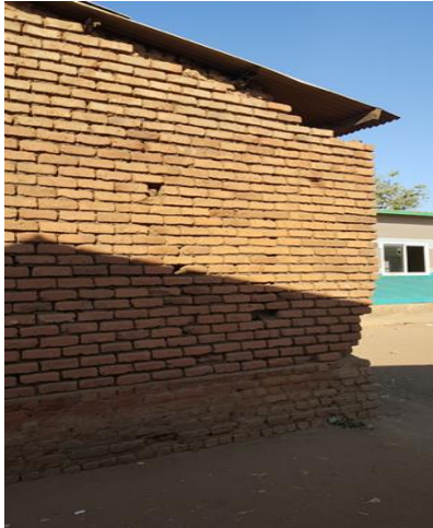
Malawi: Tsbango I Schools, failure of mortar and bricks (conventional), Image by IMC staff, 2018
