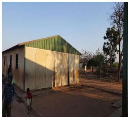
Malawi: Mvama Schol, failure of wall panels (prefab), Image by IMC staff, 2018
