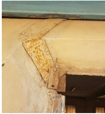
Malawi: Blantyre School, repair of wall panels (prefab), Image by IMC staff, 2018
