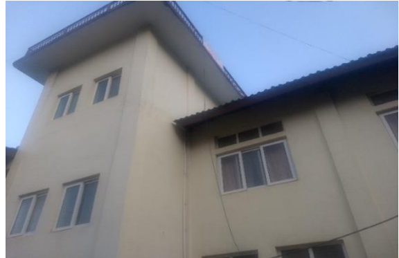
Nepal, inadequate flashing (conventional), Image by IMC staff, 2018
