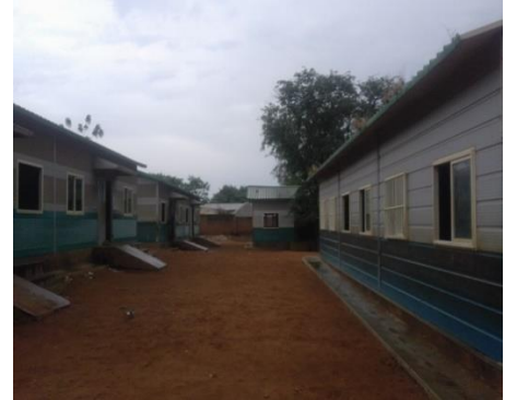
Malawi: Lilongwe School, damaged windows (prefab), Image by IMC, 2018
