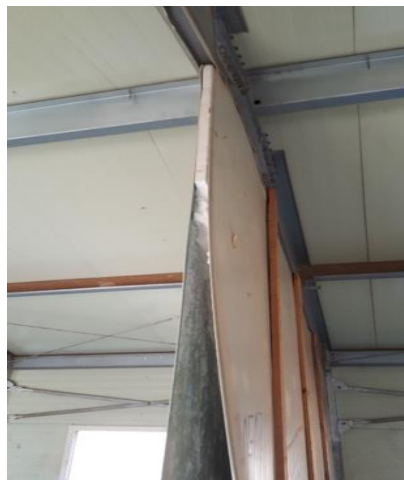
Malawi: Tsbango I Schools, partition failure, (prefab), Image by IMC staff, 2018
