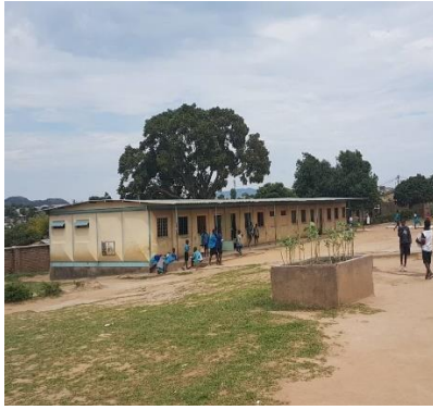
Malawi: Blantyre School, repair of wall panels (prefab), Image by IMC staff, 2018
