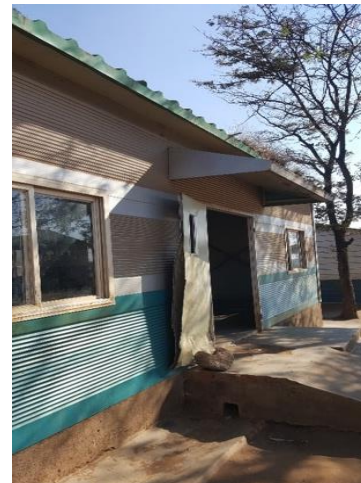
Malawi: Tsbango I Schools, malfunctioning/missing doors, (prefab), Image by IMC staff, 2018
