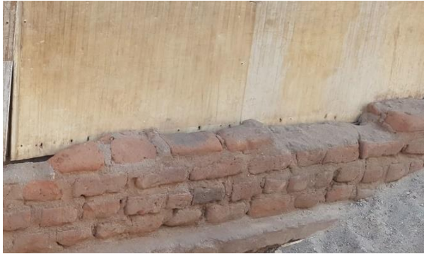
Malawi, adobe bricks used to hold back siding (prefab), Image by IMC staff, 2018
