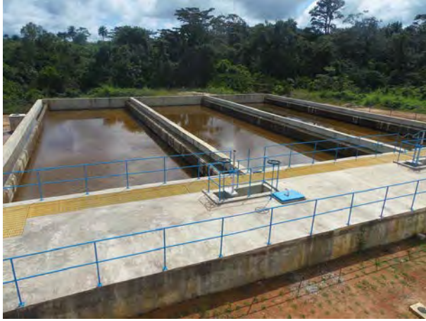
Figure 3: Slow Sand Filter at USAID's WTP in Sanniquellie.
