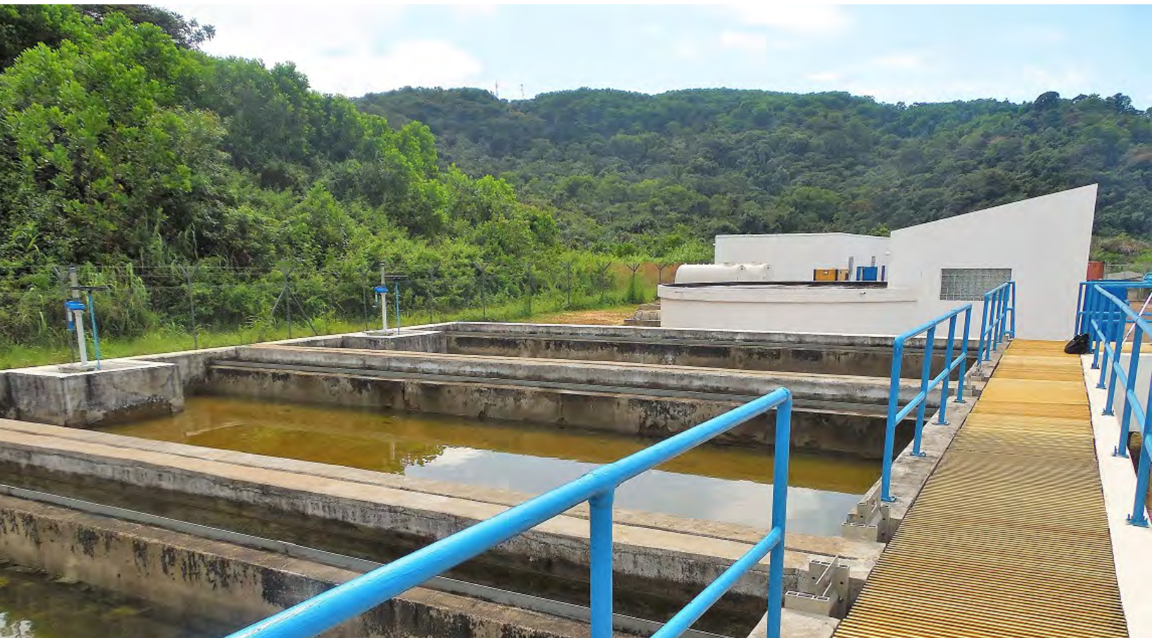
MARCO VISSER FOR SOCIAL IMPACT: ROBERTSPORT WATER TREATMENT PLANT
