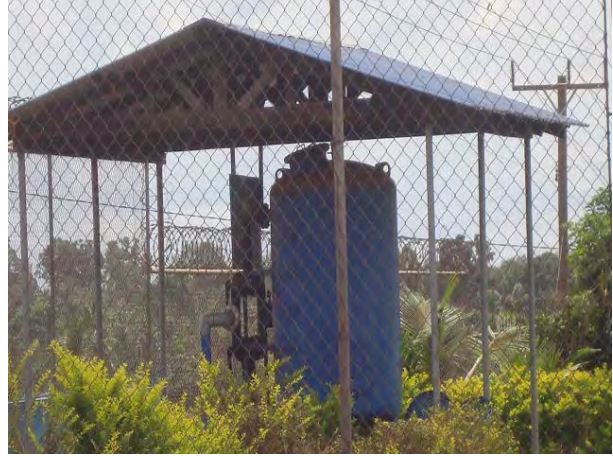
Figure 42: AfDB Water Treatment Station in Kakata.
