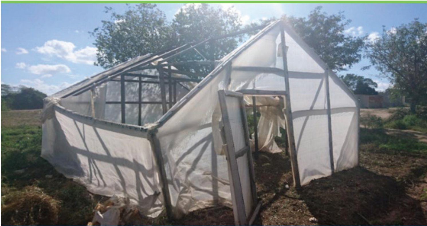
PHOTO 3. Damaged greenhouse. The greenhouse was out of use, but its owner has plans to fix it. It is not known when the greenhouse was damaged.
