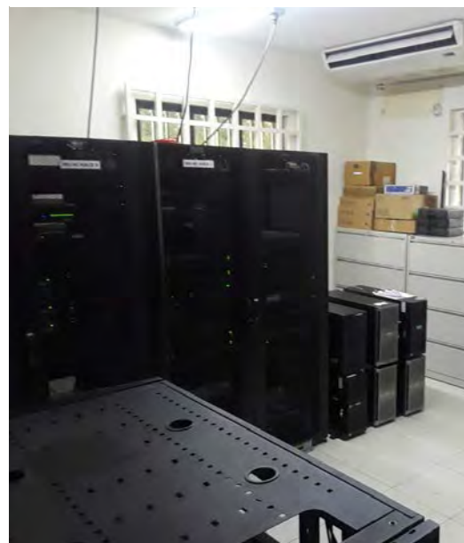
FIGURE 6. DGI CENTRAL NOC
