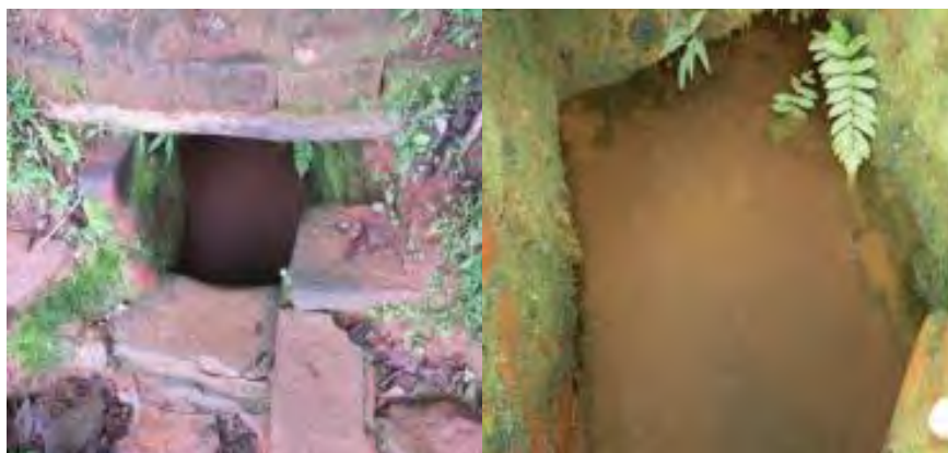
Unprotected spring in Zanapoosa
