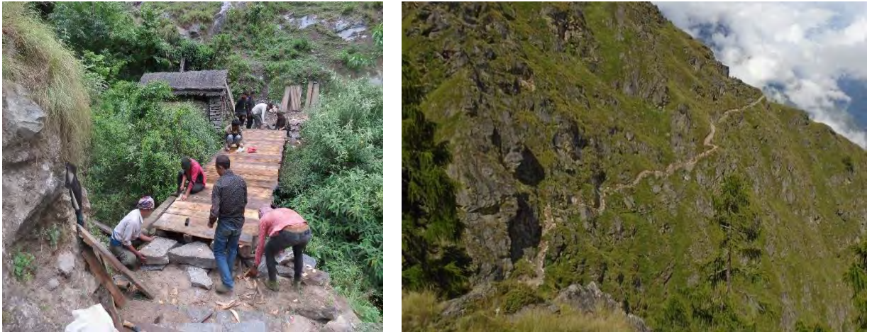
Plate 9 Bridge repair at Nawang khola, Sirdibas, and Bihi-Chumchet alternative route by NTNC © NTNC, Hariyo Ban Program (both photos)
