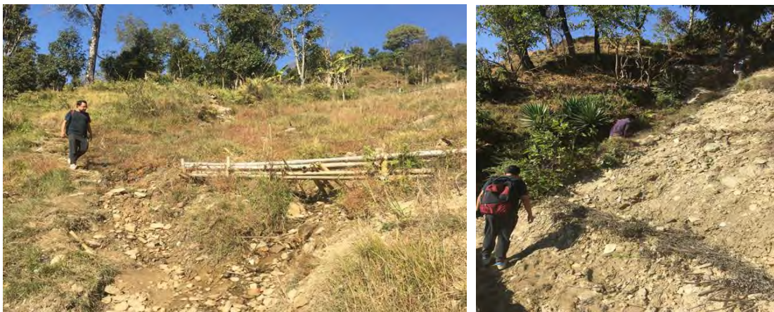
Plate 13: Field evaluation and the view of swept away crib wall
