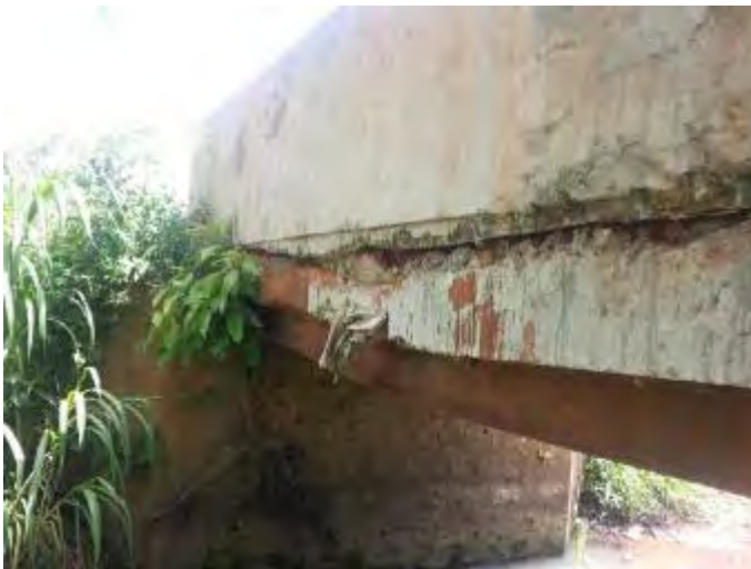
Figure 8: UNOPS should conduct a safety review of rehabilitated or new infrastructure like this bridge on Yei-Kegulu-Morobo feeder road
