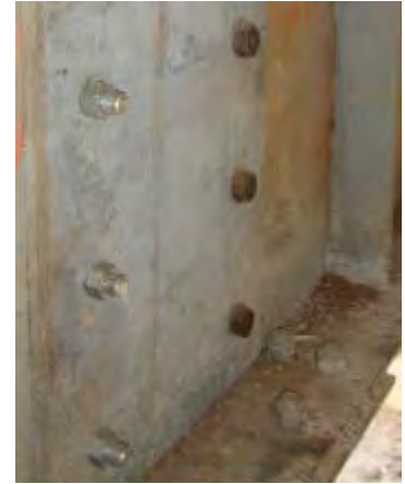
Figure 10: Different bolt types used on same structural connection at Koni River Bridge
