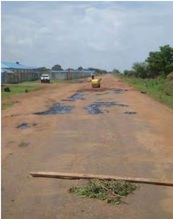
Figure 4: Defects period warranty repairs, Gumbo-Rajaf Trial Road, Central Equatoria
