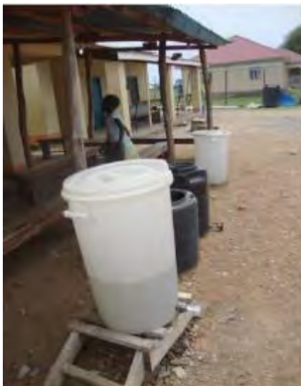
Figure 7: Current WASH facilities for main clinic building at Gurei PHCC.
